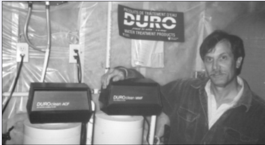
Owner: Earl Leger, Earl Leger Plumbing & Heating Ltd.
