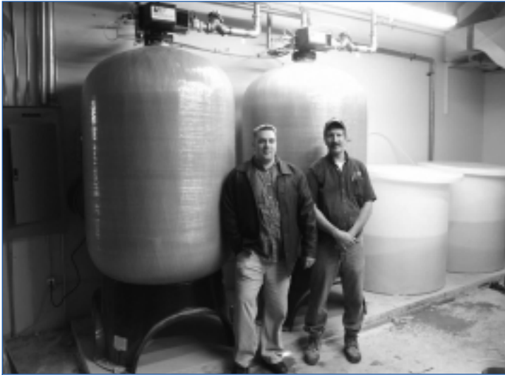
Ken Ware of Conestogo Mechanical standing to the right and Terry Morrison, Commercial Products Engineering Technologist with USF WaterGroup, are shown after initial start-up of the first set of softeners.
